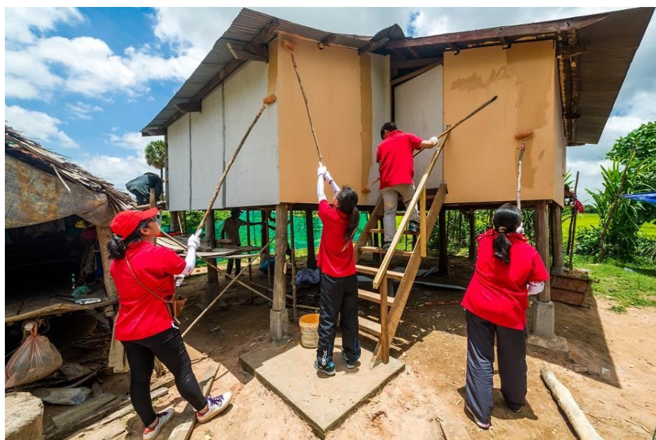
Participants of the 2016 AIA YLDP visited Cambodia to help local residents build houses.
